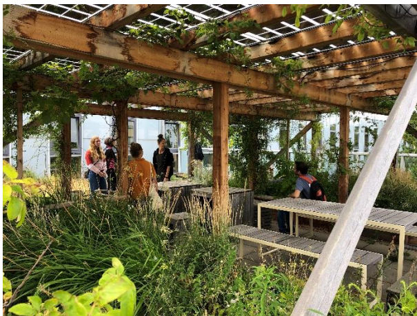
Visit to the photovoltaic system at Schwackhöfer House at the BOKU University Campus © OeAD-WVGmbH
